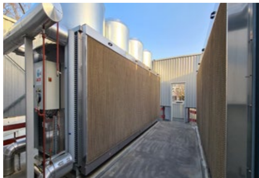
The CNRS is attempting to find sustainable solutions to renovate and maintain its research buildings and equipment. Here, we see the cooling system for the Jean Zay supercomputer. The machine's heat will be recovered and fed into the Paris-Saclay urban campus's heat and cold exchange network. © Rafael MEDEIROS / IDRIS / CNRS Photothèque
